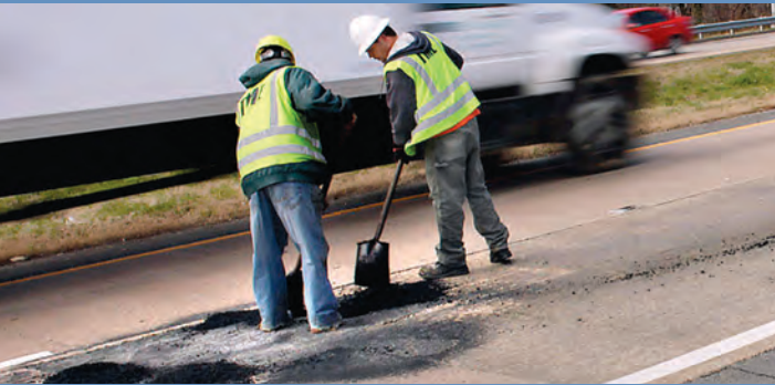
Pot Hole Repair Companies
